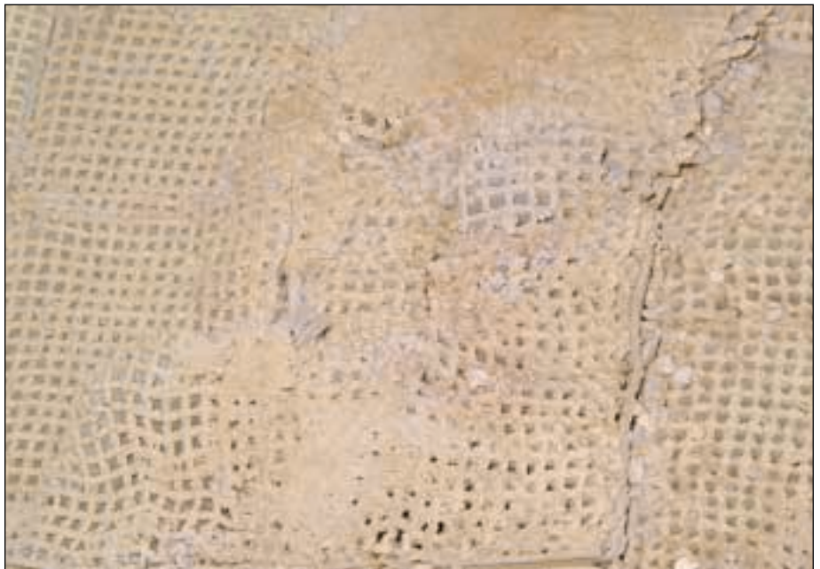
Figure 2: severely restricted airflow
